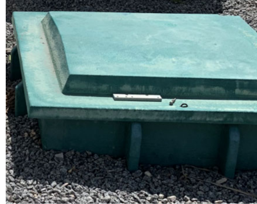
GREEN VAK PAK SURGE TANK
