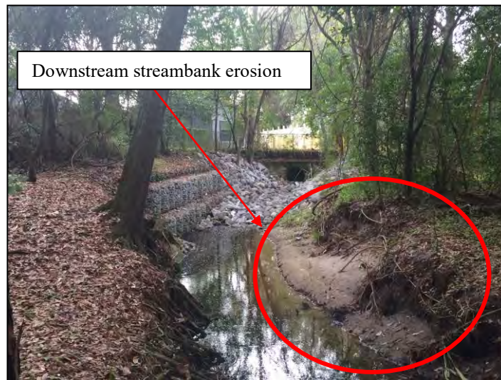
Figure 2 Evidence of streambank erosion
